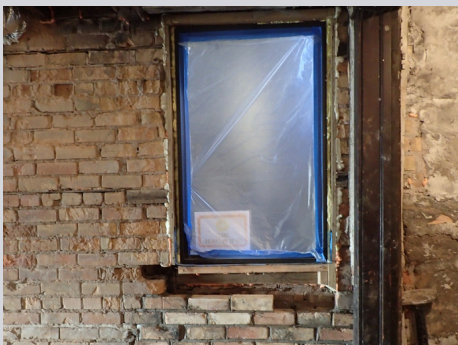
Damaged brick before restoration.
