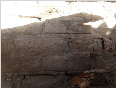
Damaged and dirty brick before restoration.
