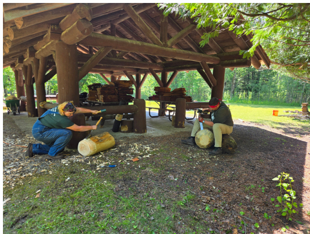
Corpsmembers stripping logs that will be used as corner pieces in the picnic area.
