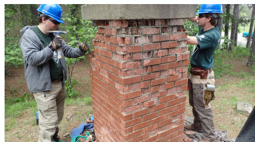
Corpsmembers repairing a brick pillar at the entrance to the Ely Cemetery.
