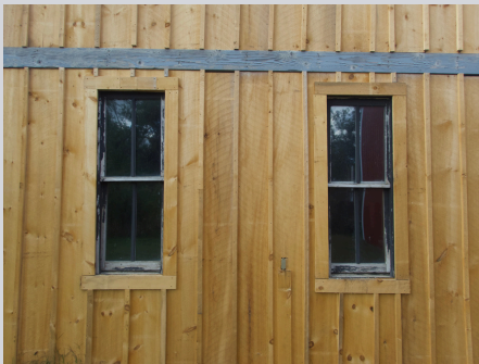
A photo of the window before repair.
