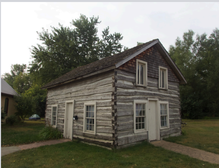
A photo of the roof before repair.
